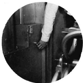
FIG. 5. Open collector drain valve.
